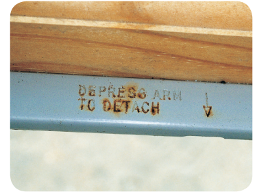
Moisture accumulation from logos, stampings, and rivet holes.
